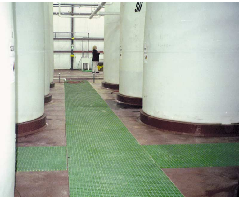
The Exide Battery Plant in Manchester, Iowa installed corrosion resistant DURAGRATE® around its tanks of sulfuric acid.
